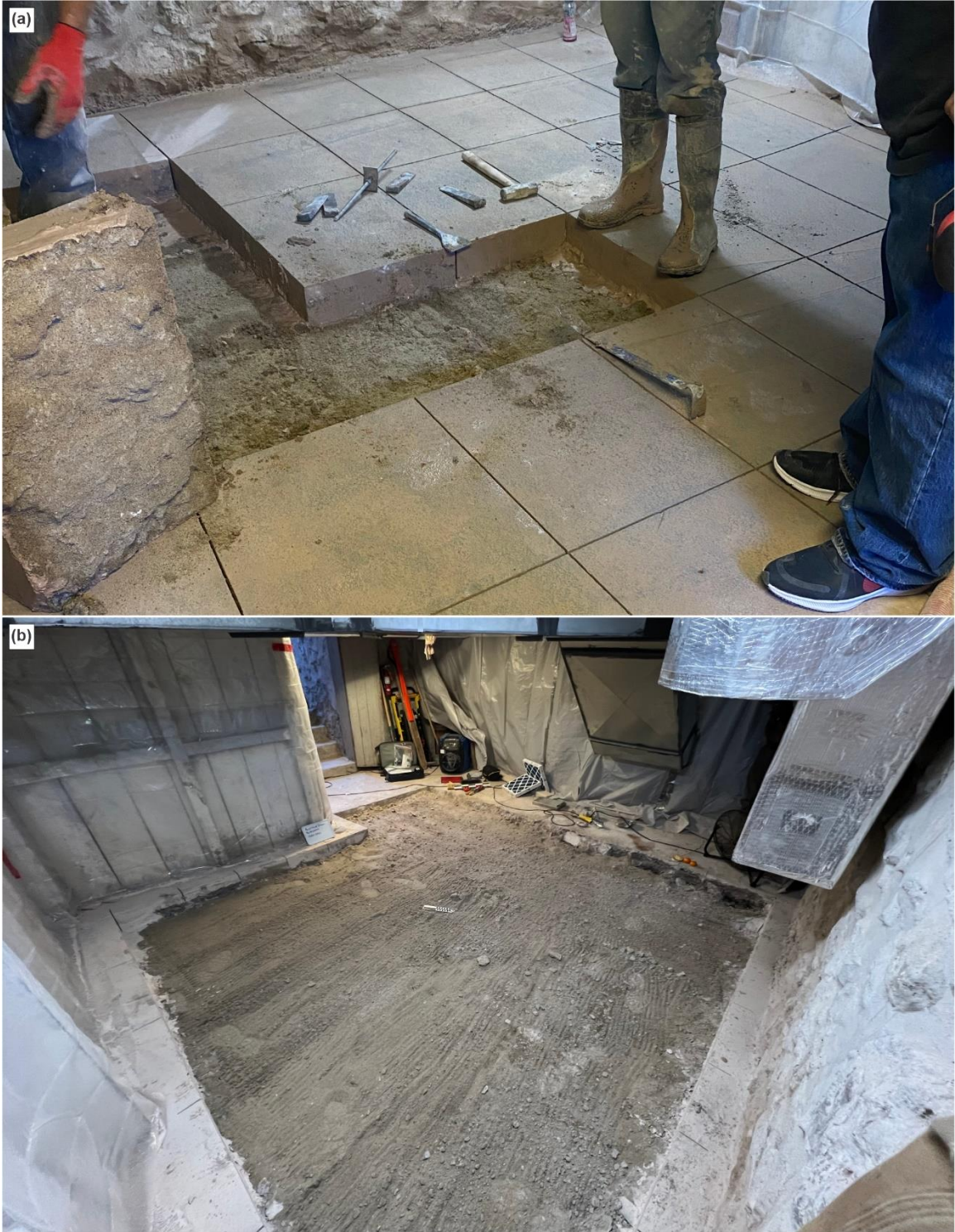
Figure 5. Concrete removal before excavation: (a) to help project what might be below, the concrete was cut into sections for removal by hand (rather than jackhammering), and (b) the concrete removed from the excavation area exposing the sandy/gravelly substrate used to level off the area before the concrete was poured (the surface was lightly raked after the concrete was removed).
